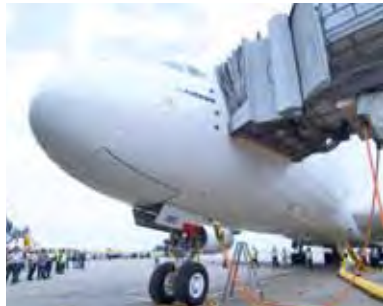
Provision of fixed ground power and pre-conditioned air systems to aircraft 為客機提供固定地面供電系統及預調空氣系統
