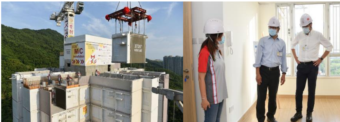
Figure 7. First Concrete MiC Construction in Hong Kong (2020) – Married quarters for the Fire Services Department at Pak Shing Kok, Tseung Kwan O Construction site (left) and Building Interior (right) 16
